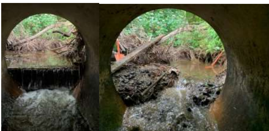
Figure 6: Fish barrier remediated in a tributary of the Waikawa Stream. Photo on the left shows prior to remediation (a drop due to a wooden board covering entrance to culvert) and photo on the right after remediation by removing the board.
